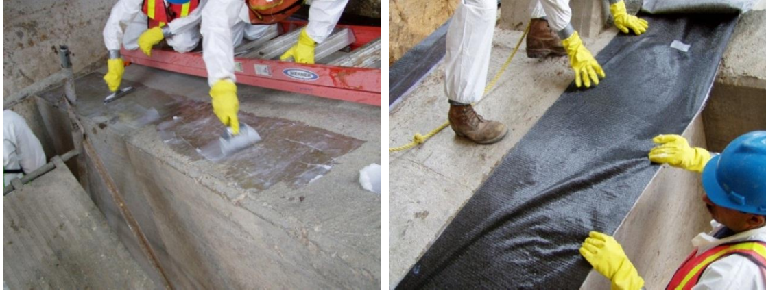
Figures 3.12 and 3.13. Fyfe’s Tyfo® S Epoxy resin (likely with glass fibers as a filler) being applied to the extrados of an arch and installation of saturated unidirectional CFRP fabric, Tyfo® SCH-41 (Mohseni, CDOT)
