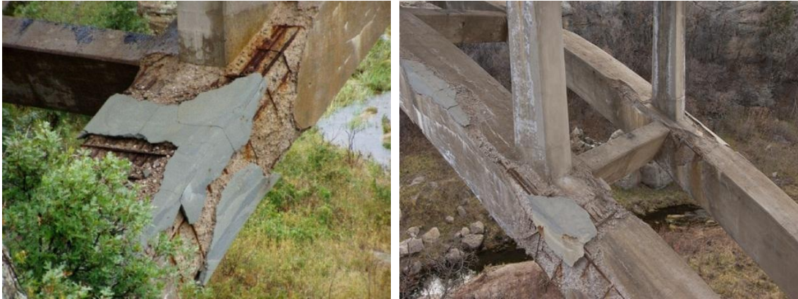
Figures 3.8 and 3.9. Concrete spalling on arch section prior to repair (Mohseni, CDOT)
