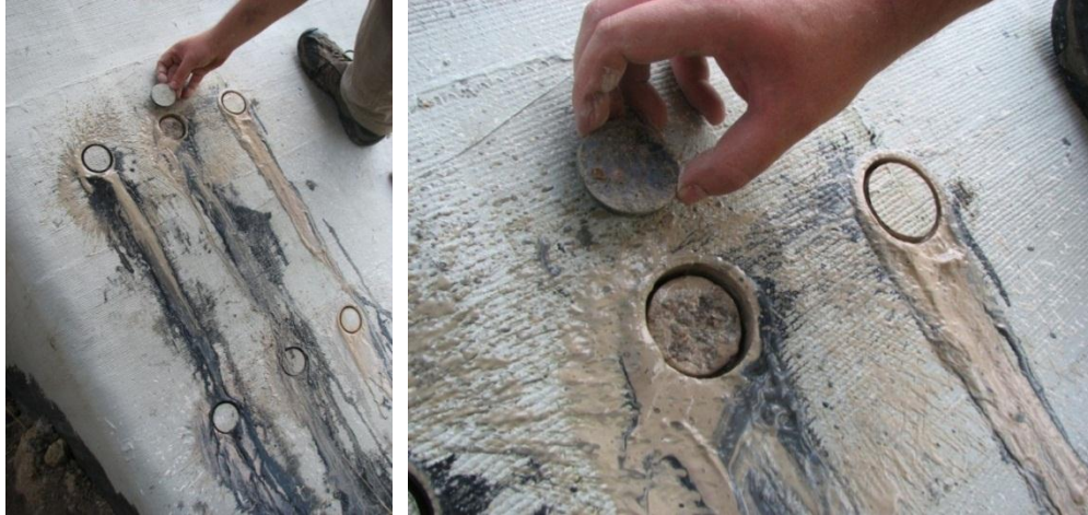
Figures 3.27 and 3.28. The core drilling location that failed due to torsional stresses during the core drilling process, bay 1NW
