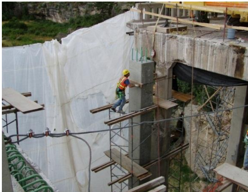
Figure 3.7. Placing the new spandrel columns adjacent to the existing columns (Mohseni, CDOT)
