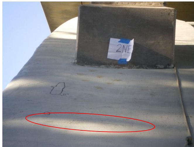
Figure 3.20. Crack identified in 2007
