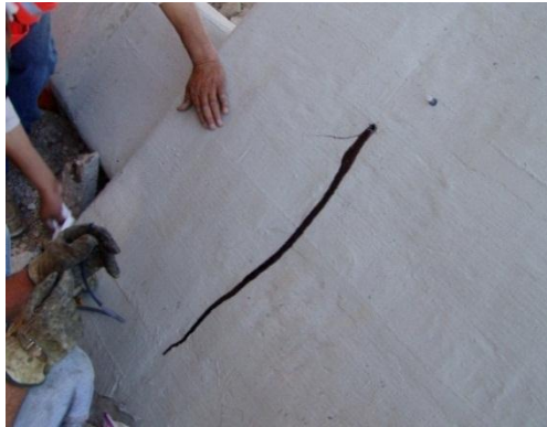
Figure 3.15. Void injected with resin during 2003 renovation (Mohseni, CDOT)
