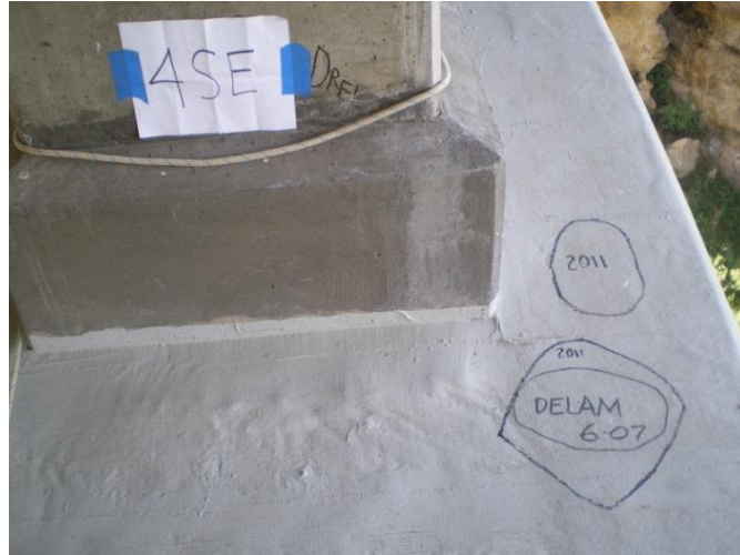
Figure 3.19. Enclosed in permanent marker are identified areas of debonded areas between the FRP and the substrate from 2011 and June, 2007. Notice in this more protected bay of the structure the markings from 2007 are more clearly visible.
