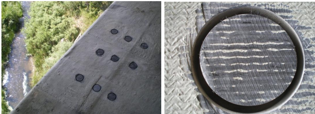
Figures 3.31 and 3.32. Prepared areas for the adhesion of aluminum pucks for pull-off tests and a close-up of a prepared surface
