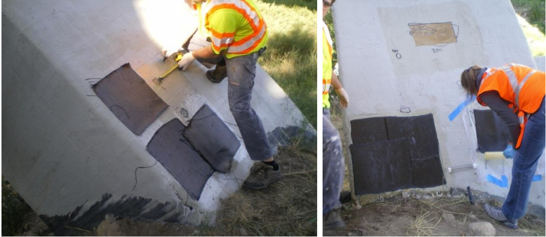
Figures 3.57 and 3.58. Allocating fabric for repair and applying the second layer of CFRP to the area of pull-off tests on the east arch
