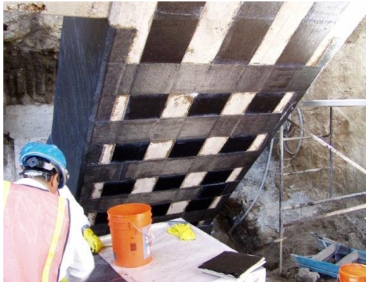
Figure 3.14. Longitudinal and transverse CFRP wraps at the base of an arch (Mohseni, CDOT)
