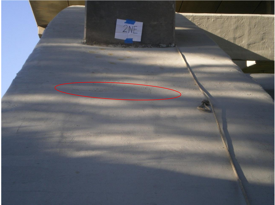
Figure A7. Bay 2NE, Crack enclosed in red oval was identified in 2007
