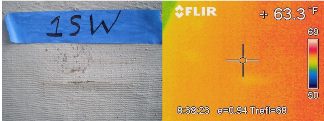
Figure A24. Photograph and thermal image of a defect found in Bay 1SW
