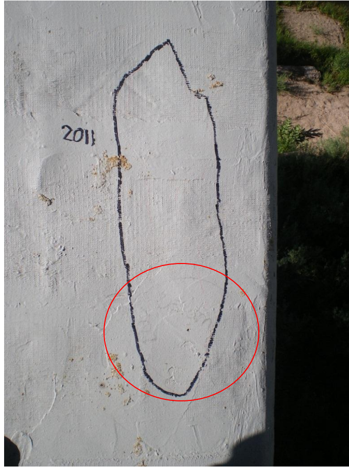
Figure A11. Enclosed in the red circle is 1 of the 2 voids found in 2007
