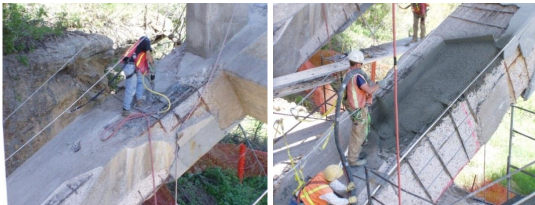
Figures 3.10 and 3.11. Removal of loose concrete using 6.8 kg (15 lbs.) jackhammer and restoring the cross section with shotcrete (Mohseni, CDOT)
