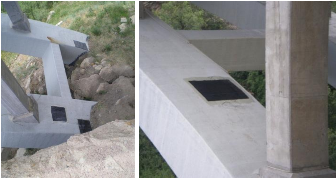
Figures 3.59 and 3.60. The repaired sections on the north end of the arches
