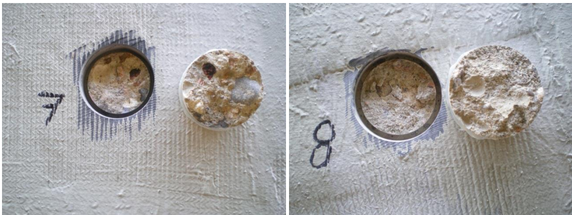
Figures B22 and B23. Test No.25 and Test No.26, note very weak bond strength (poorly mixed concrete?)
