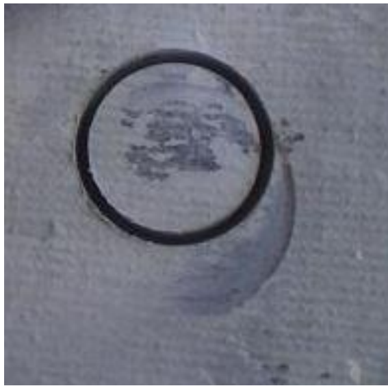
Figure 3.25. Damage caused by core bit without the use of the jig
