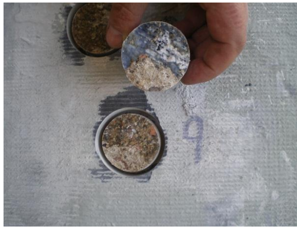
Figure B8. Test No.9, weak bond strength
