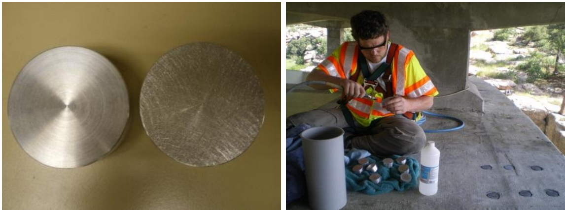
Figures 3.33 and 3.34. Aluminum pucks before and after sanding with 40 grit sandpaper and preparing the aluminum pucks way up high on the arch
