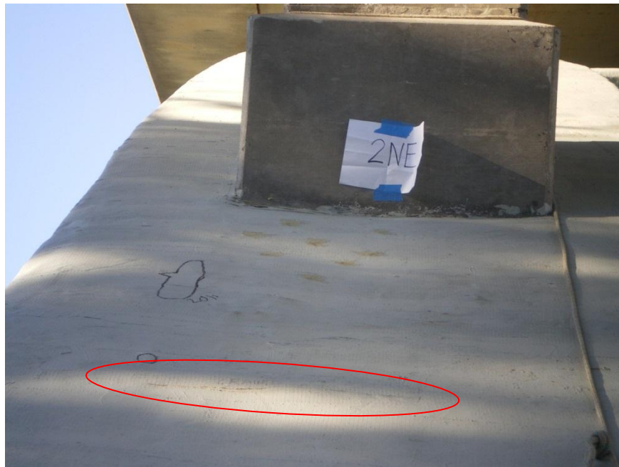
Figure A8. Previously identified in 2007, a crack enclosed in the red oval, no debonding at the location of the crack
